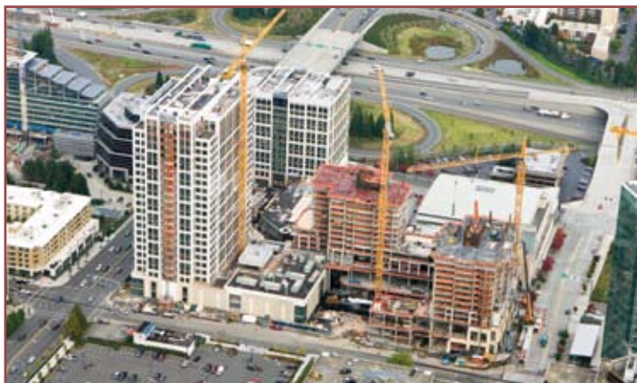
Aerial view of the four and a half acre construction site for The Bravern.
