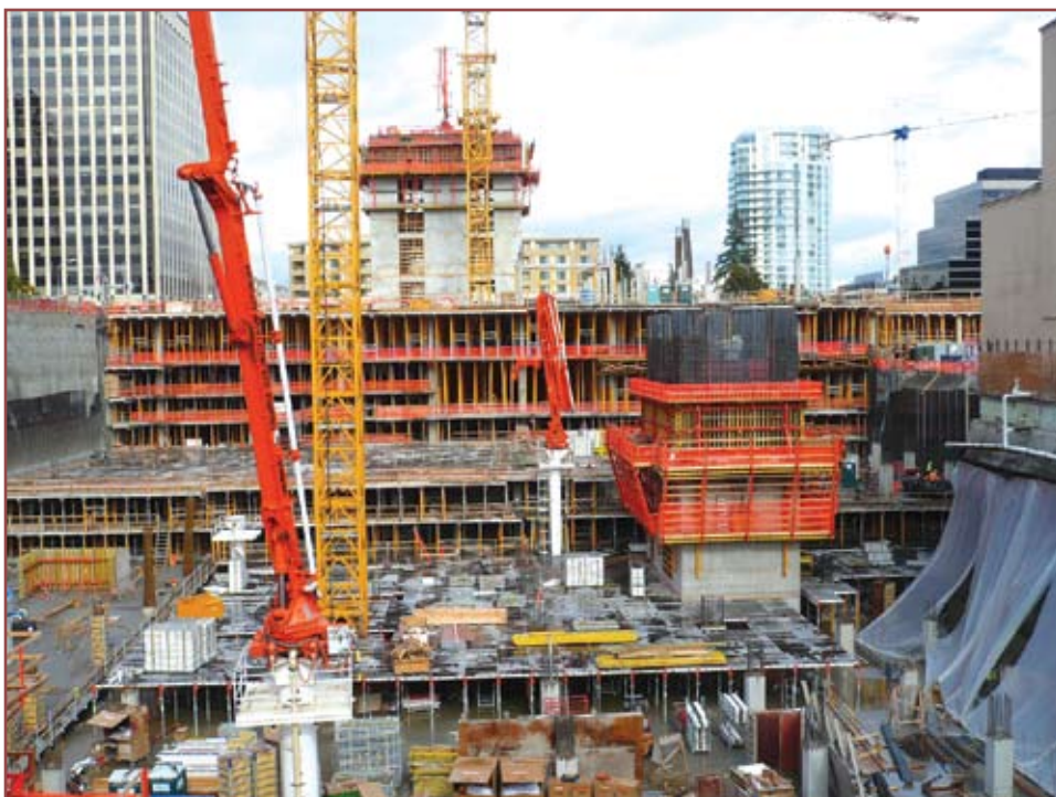
Early photo showing the various construction stages of the seven below-grade parking levels.
